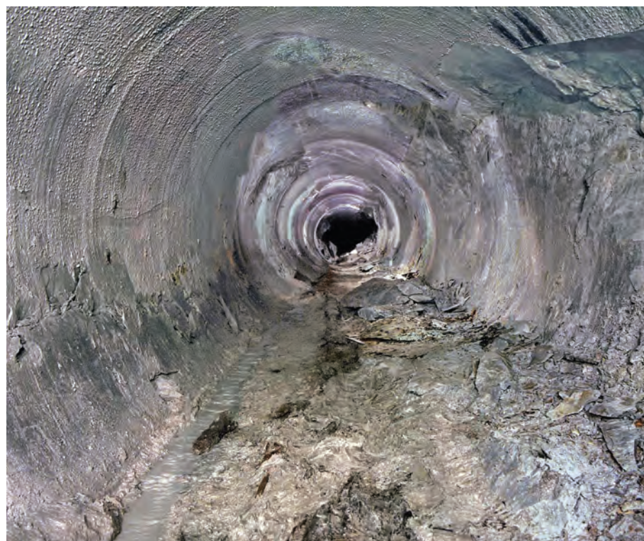
A section of Watkin's attempt to build a Channel Tunnel can still be seen at Folkestone Warren. Photo Nick Catford
